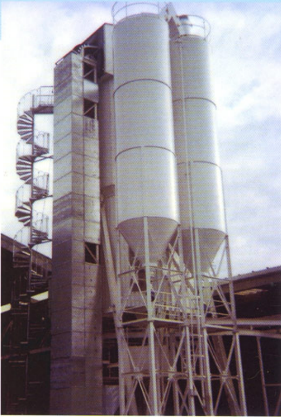
TEB conveyor with distributor to the cells of the bin with 25 m. of height.
