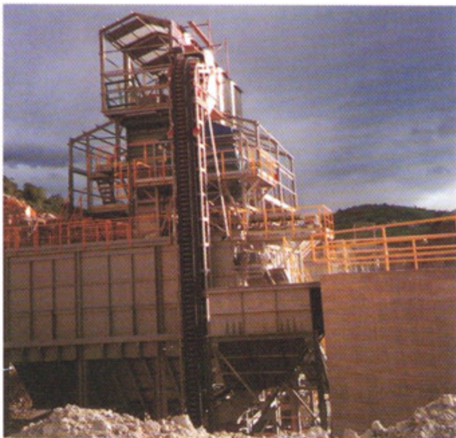
TEB conveyor at treatment of aggregates installation.
