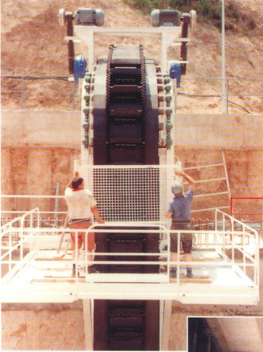
Detail of unloading header with maintenance platform.
