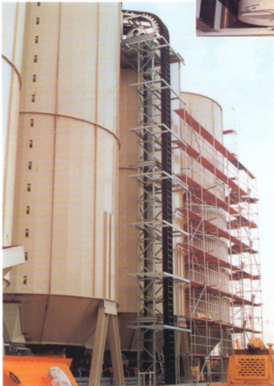
TEB conveyor for filling of several products in storage bins.
